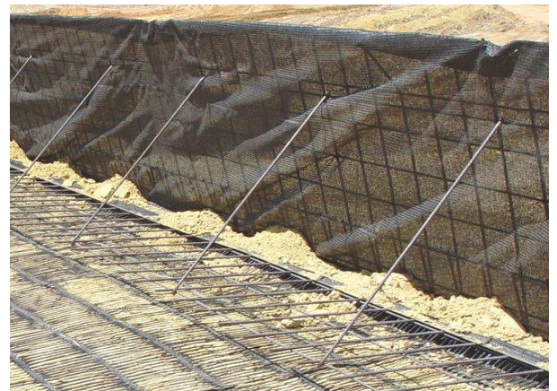
Figure 3 Steel brace bars fixed in position to maintain the required 70° face angle
